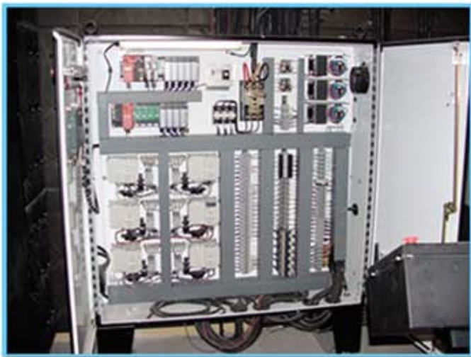
AET UL 508A CONTROL CABINET
